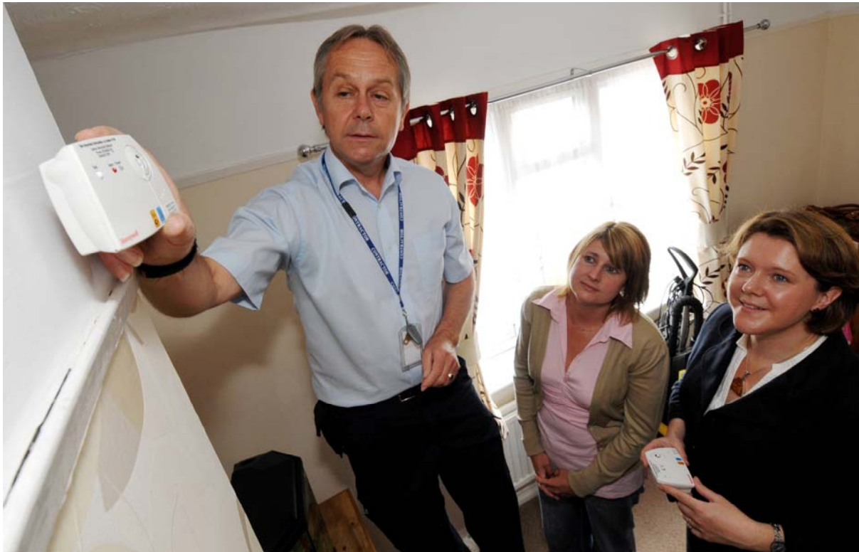
CHS contractor fits carbon monoxide detector watched by Maria Miller MP (far right) and resident, Mrs Davis
